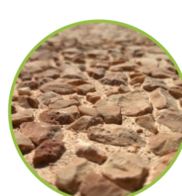
Deep exposure. Exposure depth approx. 4 mm
