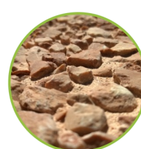
Deep exposure. Exposure depth approx. 6 mm
